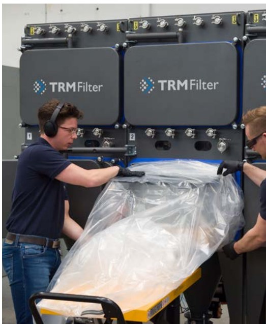
Primary filter replacement with protective bag
